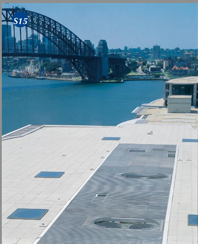
The Quay, Sydney, NSW, HA503 and HC503 grating forming a non-trafficable vision screen over the irregular plant room and ducting equipment.
